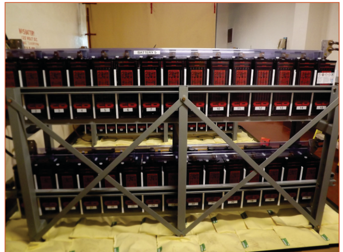
One of the battery racks at RH Saunders
