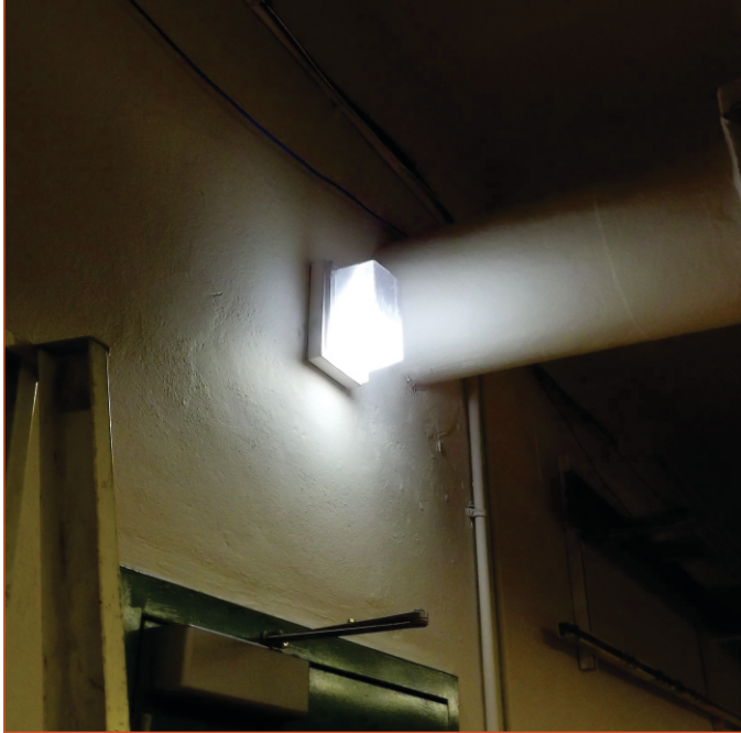
Emergency-Powered LED Lighting In-Action
